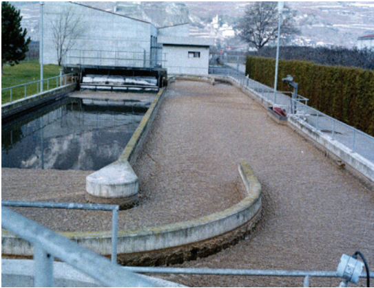
Fig. 2. Before treatment, with heavy FOG.
